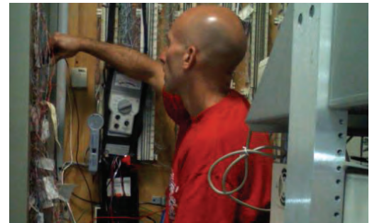
Even the equipment is probably glad to have an experienced union member back to do T1 maintenance at Neptune Ave. in Brooklyn
